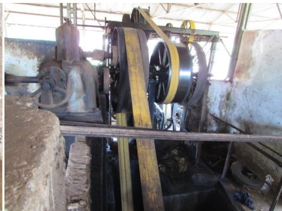
Figure 4: AMHP scheme providing mechanical drive in a sisal plantation in Tanzania.
