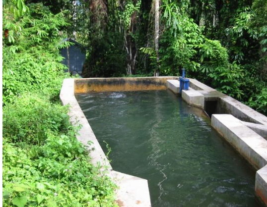
Figure 33: Forebay tank with spillway, trash rack (submerged) and flushing gate.
