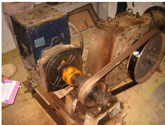
Figure 48: A poorly kept powerhouse & E/M equipment. This indicates a poorly maintained scheme overall.
