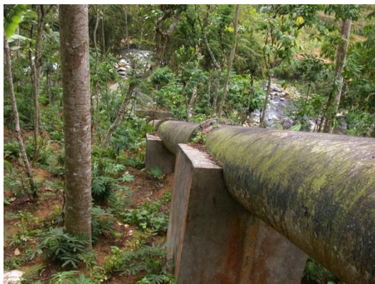
Figure 18: Poorly maintained penstock pipe. Over time lack of protection and contact with soil / vegetation will lead to corrosion.
