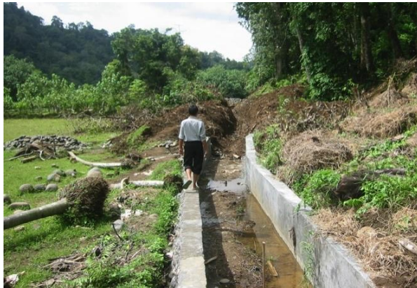
Figure 9: A headrace channel blocked due to a landslide.
