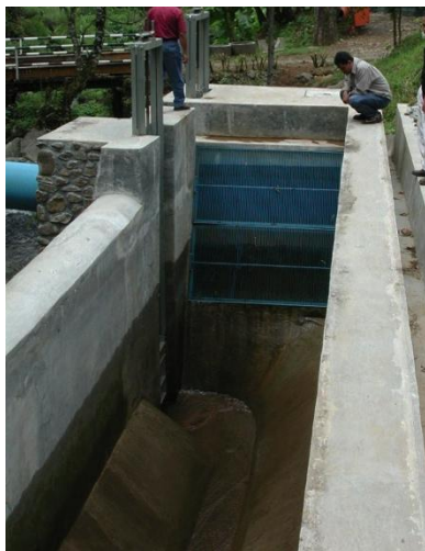
Figure 36: View of trash rack positioned in settling basin.
