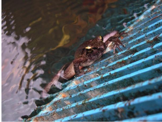
Figure 38: A good example of a properly made trash rack from 1cm steel flat bar in operation – keeping unwanted visitors out!
