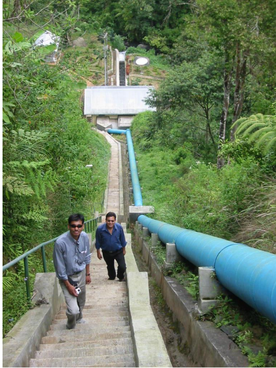
Figure 40: Typical above ground spiral welded steel penstock pipe. Anchor blocks and supports clearly visible.
