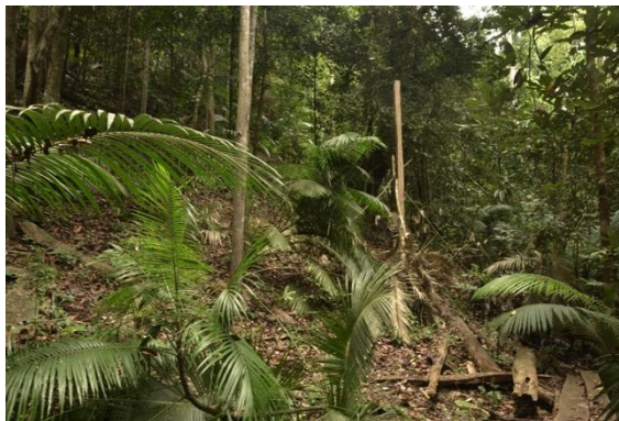
Figure 52: Erection of transmission line in densely vegetated forest. Regular cutting back of vegetation will be necessary.
