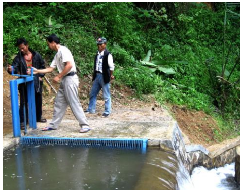
Figure 13: Settling basin being flushed
