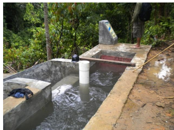
Figure 100: Water spilling over the side spillway. Flushing is achieved by removing the white PVC pipe visible in the center of the tank. This functions as a flushing pipe plug.
