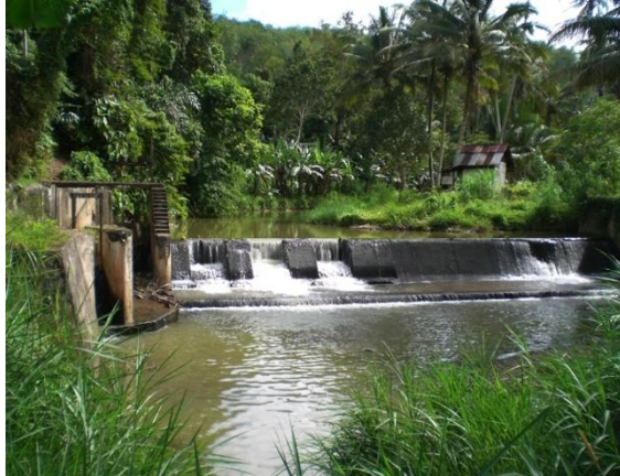
Figure 23: Less conventional weir structure. The weir is partly concrete and partly created with stop logs. This enables thorough flushing upstream of the weir.
