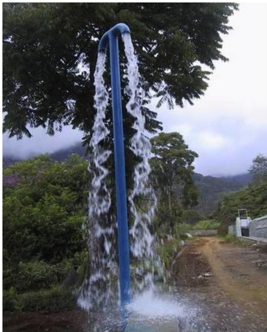
Figure 49: Ventilation / breather pipe at the upper end of the penstock enabling air to exit and enter the pipe during filling and emptying.
