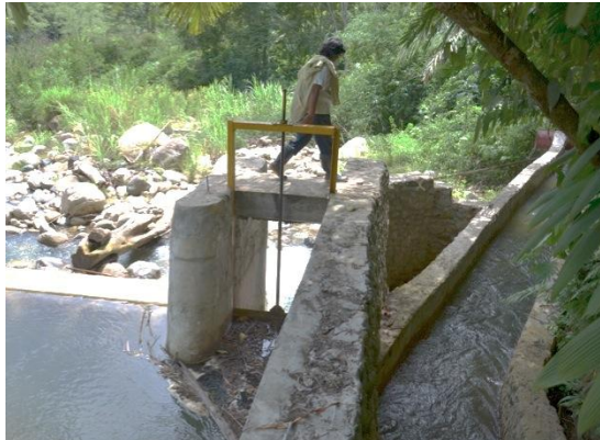
Figure 103: A submerged orifice intake. Floating debris can be seen congregating above the sluice gate but not disturbing the clean flow entering the channel.
