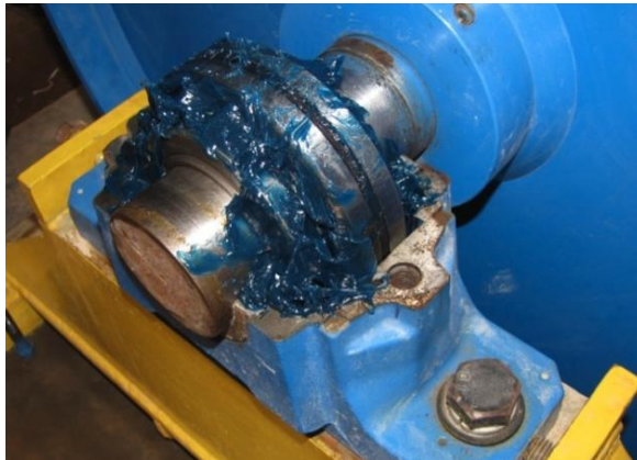
Figure 24: View of plummer block bearing with the top cover removed.
