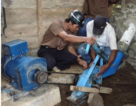
Figure 42: Low cost brush type synchronous generator on a 5 kW MHP
