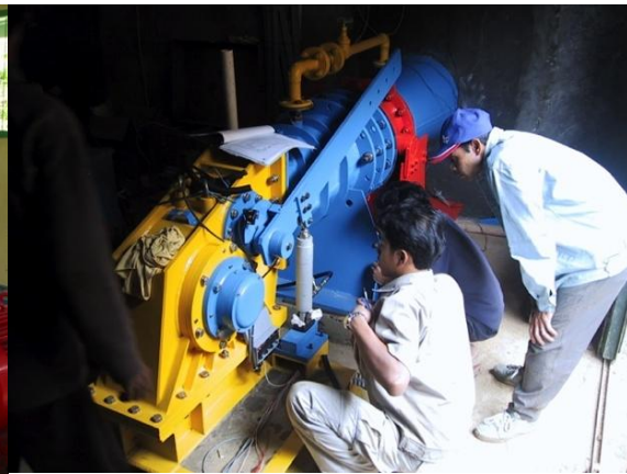
Figure 76: Example of a flow control device. The guide vane is adjusted by the small hydraulic ram visible that is controlled by a PLC based intelligent control system.
