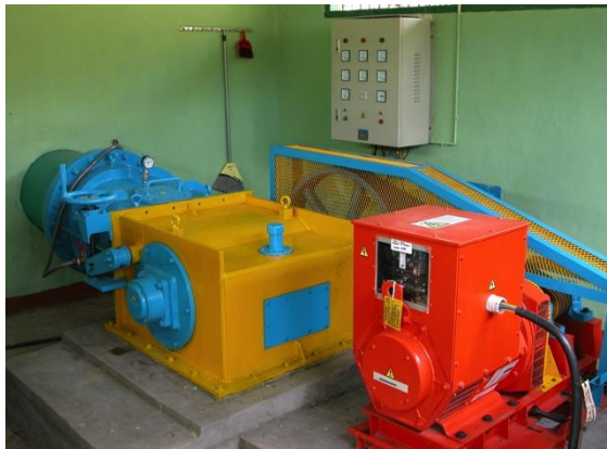
Figure 57: Typical cross flow turbine installation.
