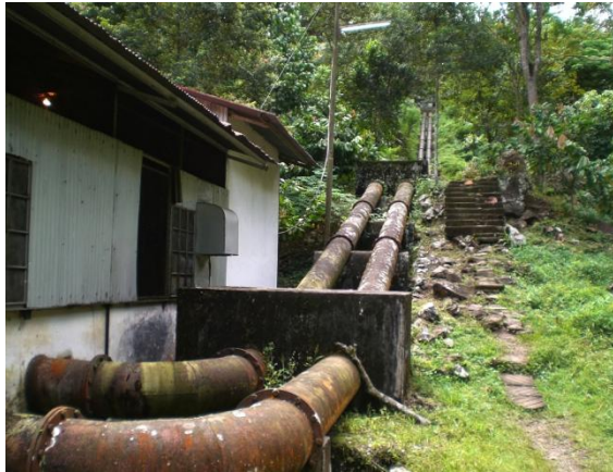
Figure 45: Twin steel penstock pipes and anchor blocks before entry into the powerhouse.
