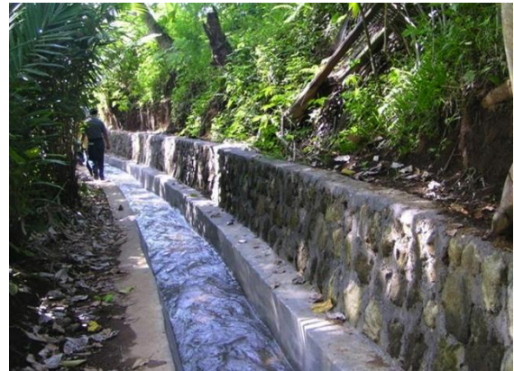
Figure 10: Construction of a retaining wall along a section of the headrace has stabilized and reduced risk of landslide on this headrace channel.
