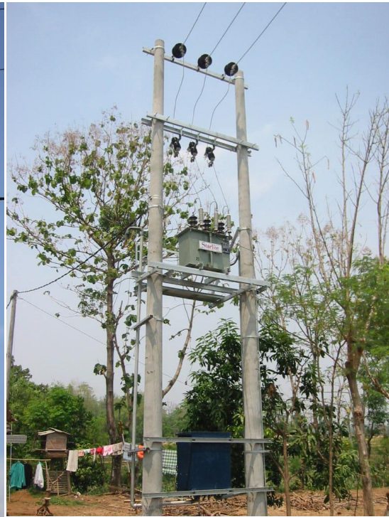
Figure 86: Step-up transformers must be positioned at a safe height above ground as in the picture or protected with a safety cage.
