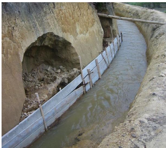
Figure 15: Damage of an unlined earth channel.
