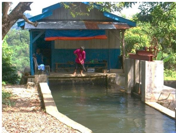
Figure 101: Cleaning the trash rack at the forebay. This is a grid-connected scheme therefore no water is spilling over the spillway.
