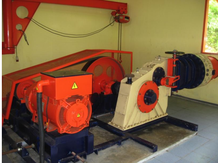
Figure 74: Synchronous generator connected via a flat belt drive to a cross flow turbine.
