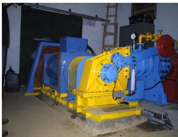
Figure 67: Shaft-to-shaft direct drive transmission. In this installation a flywheel is positioned on the far end of the generator.
