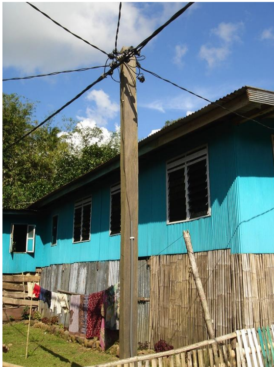
Figure 81: Example of a typical timber cable pole.
