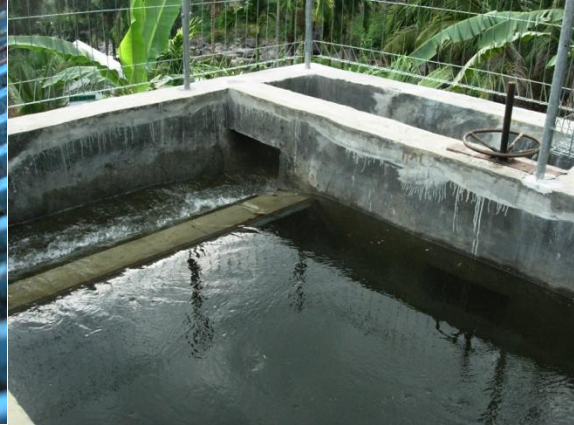
Figure 39: Submerged trash rack in forebay. A self-cleaning effect is created with the excess flow taking floating debris over the spillway.
