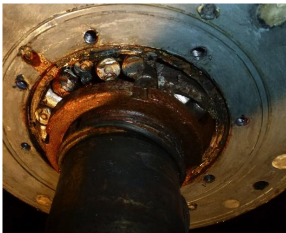
Figure 7: Total bearing failure with expensive consequences. Signs of vibration were ignored resulting in total failure and a blocked runner.
