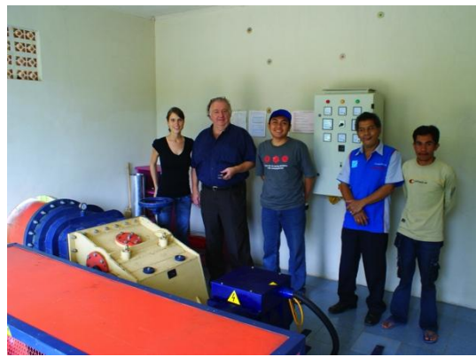
Figure 49: A well managed powerhouse. Clean and tidy after 10 years of operation!
