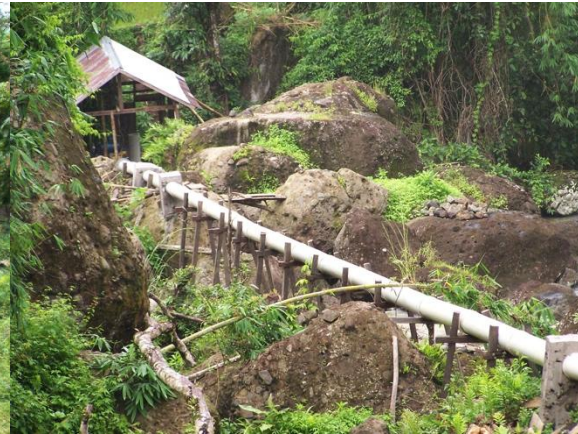
Figure 46: PVC penstock pipe installed on a low cost community based MHP.
