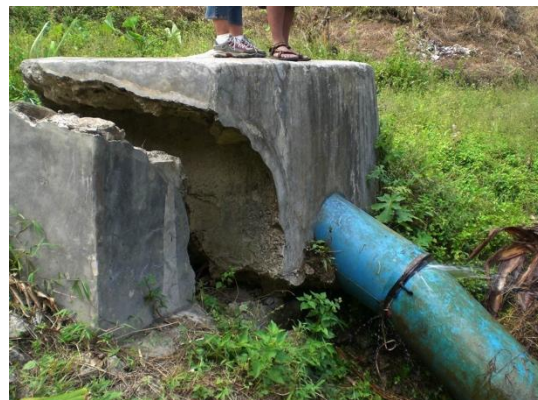
Figure 6: Severley damaged anchor block. If not repaired this could lead to more serious damage of the penstock, powerhouse etc.
