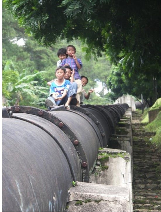
Figure 41: Flanged cast iron penstock pipe suspended above ground on concrete supports.
