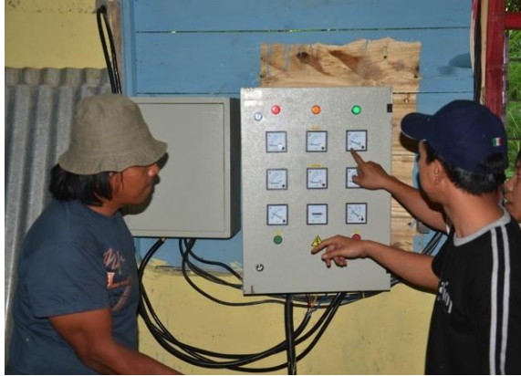
Figure 105: Checking operational parameters voltage, frequency and consumer load and ballast load.
