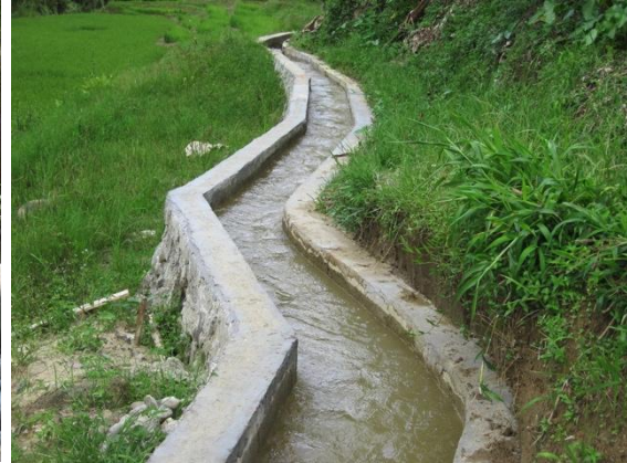
Figure 94: Regular inspection of the headrace channel should be made for damage or excessive leakage.
