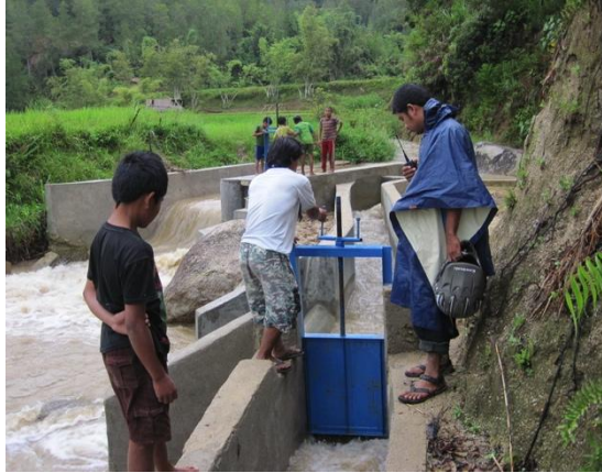
Figure 95: Opening the gate at the intake allowing flow to enter the headrace channel.
