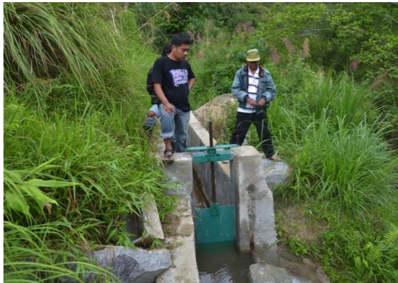
Figure 107: Headrace access gate at the intake in the closed position.
