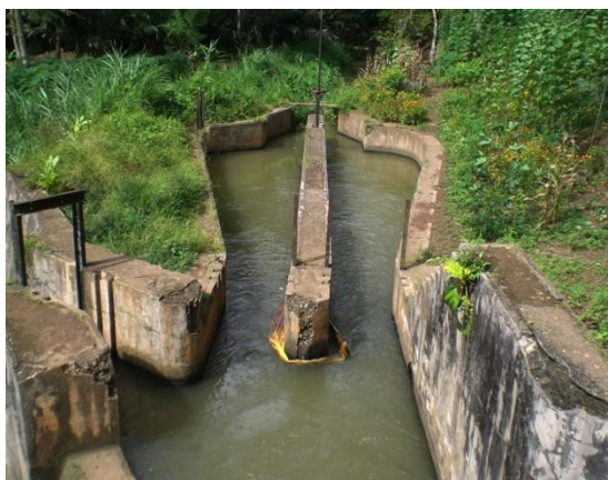
Figure 25: Parallel settling basins located immediately after the intake.
