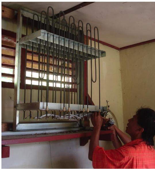
Figure 46: Air heater ballast load suspended in the powerhouse with proper ventilation.
