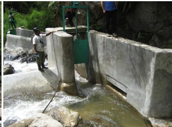
Figure 22: Weir and intake view from slightly upstream. The intake orifice is visible just above the water level.
