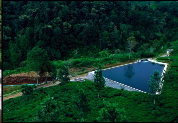
Figure 34: Large forebay / storage tank enabling the plant to supply power in excess of stream flow capacity for limited (peak load) periods.
