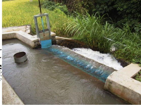
Figure 20: Drop intake transition from open channel to underground pipe.
