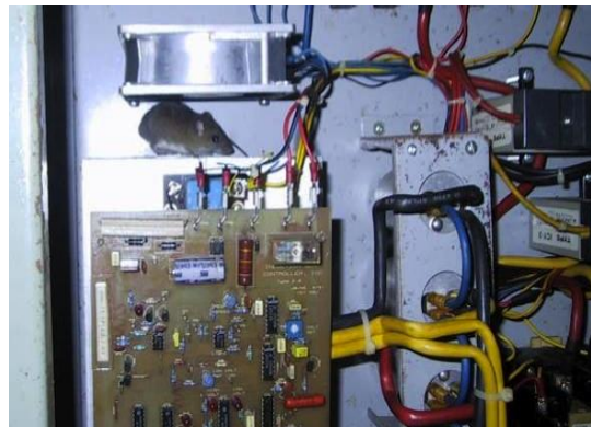
Figure 45: Mice and other small animals as seen here are attracted to the cubicle heat. They must be kept out to avoid them eating cables.
