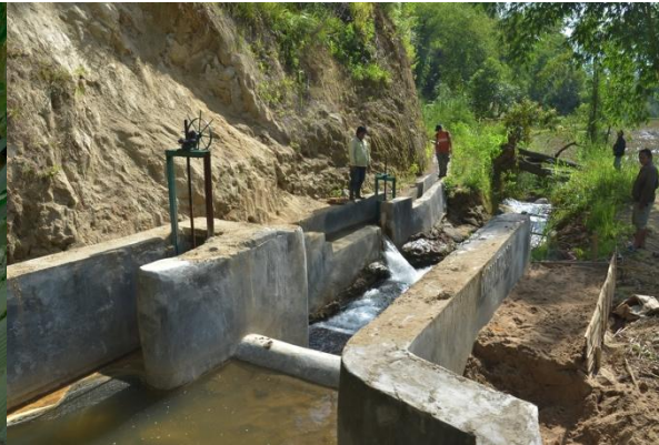
Figure 104: Intake on a small river. The flow is entering the channel via a submerged orifice. Gate into headrace is closed therefore flow is spilling back to the source.
