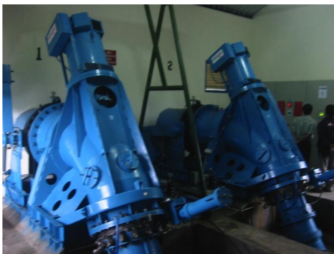
Figure 61: Locally manufactured twin propeller turbines operating on a low head scheme. The guide vanes (visible) are adjusted by a flow control device.
