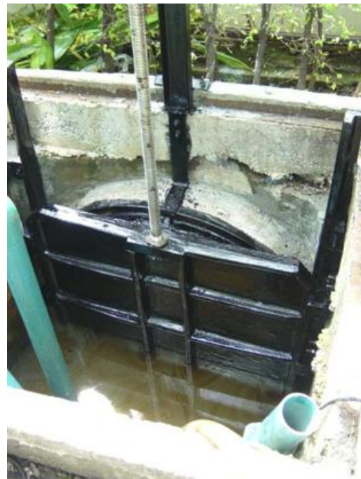
Figure 50: Typical penstock valve / gate positioned in the forebay.
