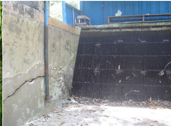
Figure 4: Cracked forebay tank as a result of an earthquake.
