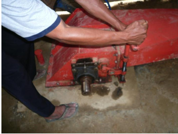
Figure 89: Ensuring the turbine guide vane / flow valve is fully closed.
