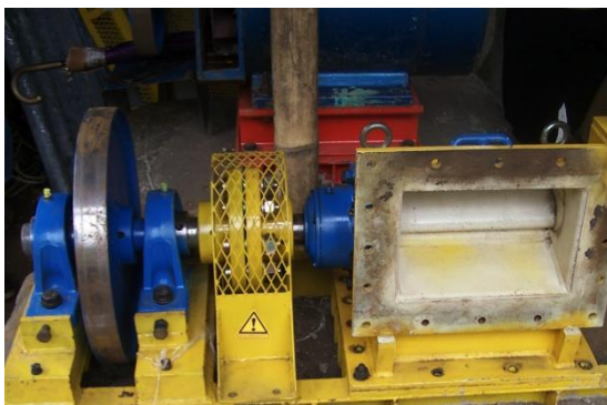
Figure 36: Flat belt transmission arrangement showing turbine, pulley, plummer block bearings and flexible coupling with guard.
