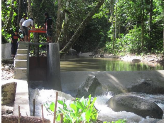
Figure 93: Periodic flushing at the intake is required. This is particularly important after large floods.
