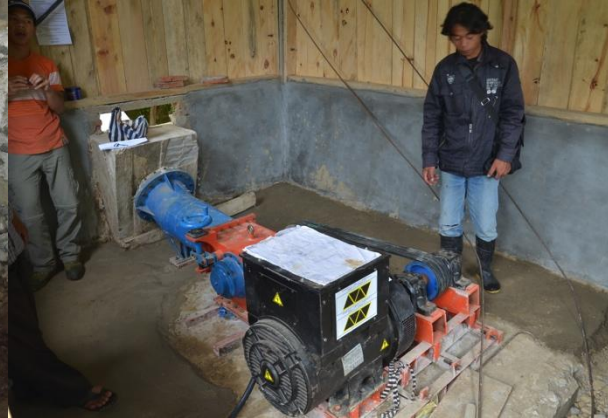
Figure 43: Brushless synchronous generator driven by a cross flow turbine.
