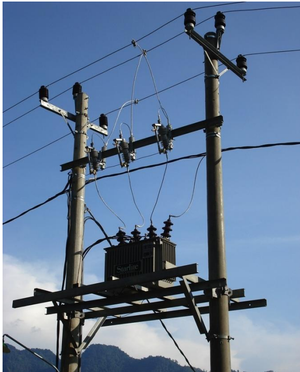
Figure 85: Typical step-up / down transformer. The medium voltage lines are suspended on the top of the poles with the insulated low voltage cable below.
