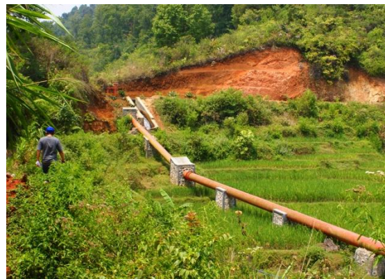
Figure 19: A properly maintained penstock kept free from contact with other elements and regularly painted.
