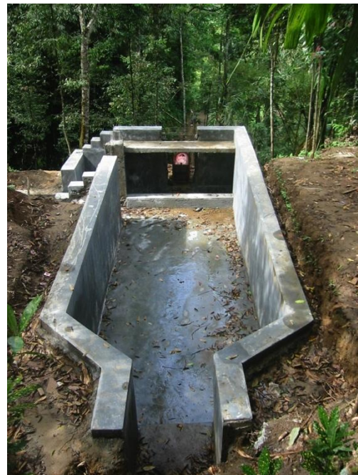
Figure 28: Recently constructed combined forebay / settling basin for a micro hydropower installation.
